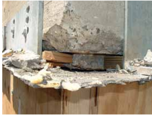
Exploratory removal of precast concrete repair panels. Note steel lintel angles and damage to original, underlying concrete spandrel
