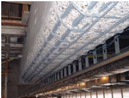
Interior beam cut back to treat reinforcement and prepare surface for concrete repair overlay
