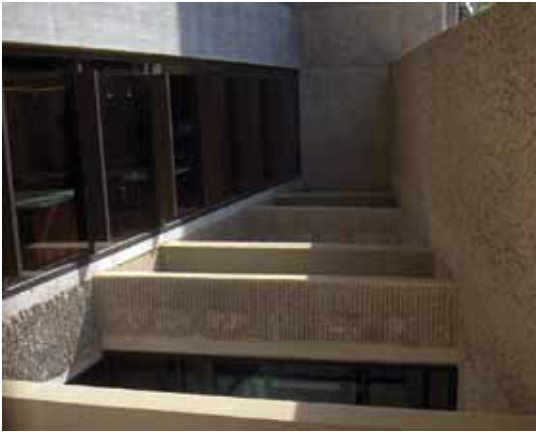
Roof coverings were removed, windows replaced, and concrete reconstructed to recreate the innovative "light wells" Rudolph originally designed
