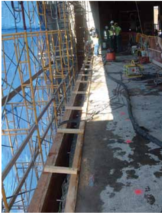
Spandrel rehabilitation in progress. Note narrow depth and wide span of repair area
