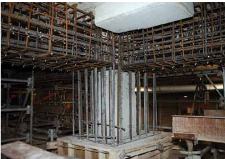
Example of congested reinforcing steel beam-column intersection. The flowability of SCC allowed the concrete around the tight reinforcing steel
