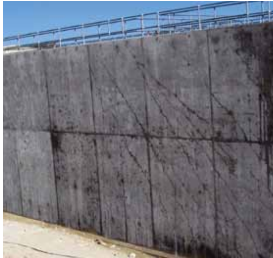
Extensive visible cracking in concrete walls
