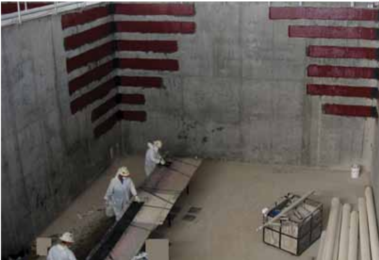
Saturating station in a single cell
