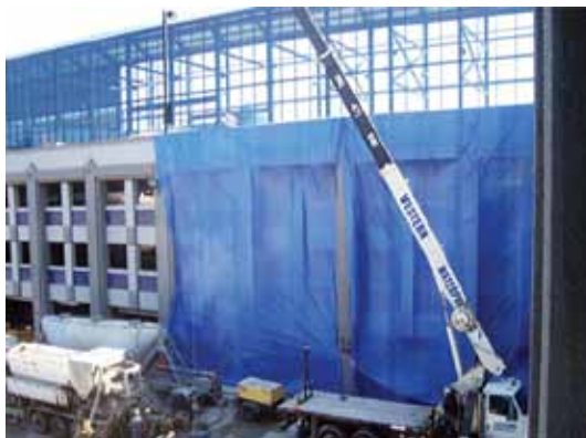
Special steps were taken during surface grinding to minimize dust spread by using tarps
