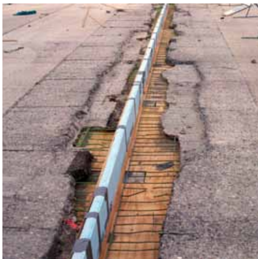
Structural repairs to the concrete tees were completed before the overlay and deck coating were installed
