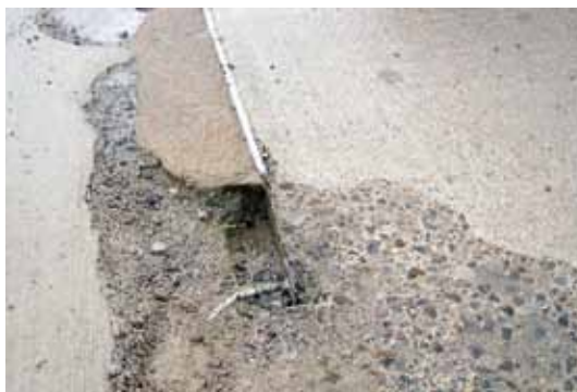
Significant failure of connectors causing movement of double-tee elements throughout the structure
