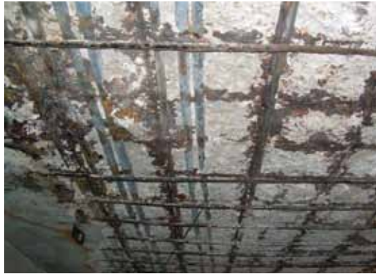
Underside of wet labs show spalling and steel corrosion
