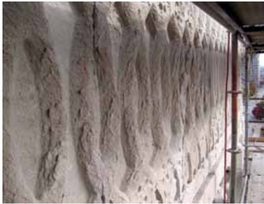
Fig. 2: Surface deterioration of carved elements
