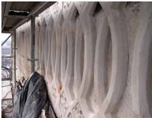
Fig. 3: Same area of carvings after patching repairs
