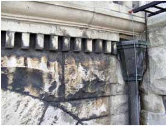
Fig. 5: Heavy gypsum crusts resistant to water spray and chemical cleaning
