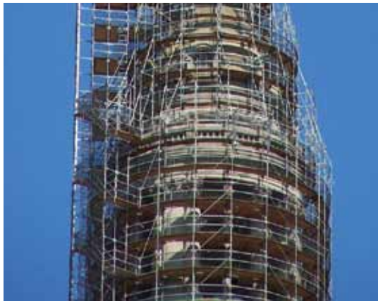
Scaffolding around the entire 37th to 52nd floors allowed engineers to inspect every square foot (meter) of the façade
