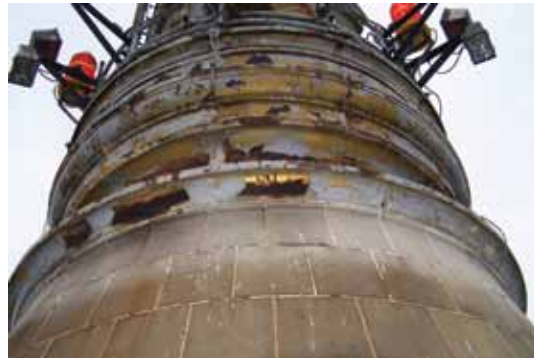
Cracked and rusted cast-iron cornices were replaced with new steel, duplicating the shape of the original
