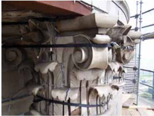
Falling pieces of terra cotta needed to be secured with straps
