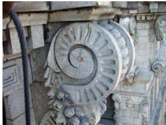
Fractured terra cotta
