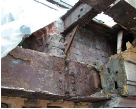
Corroded steel and cornice framing
