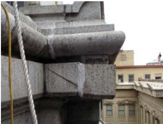
Fractured and dislodged terra cotta
