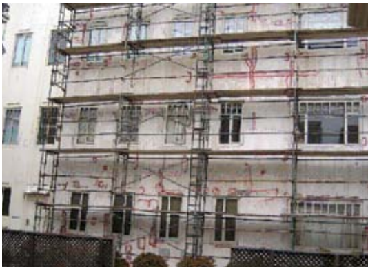
Mockup phase, coating removed, and delamination and cracks identified
