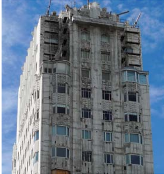
North façade with coating removed and crack and concrete repair in progress
