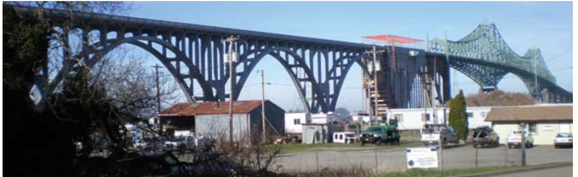
South end of the bridge. Enclosure is visible right before the steel midspan. Scope of work was to repair the South end, a 4-year project
