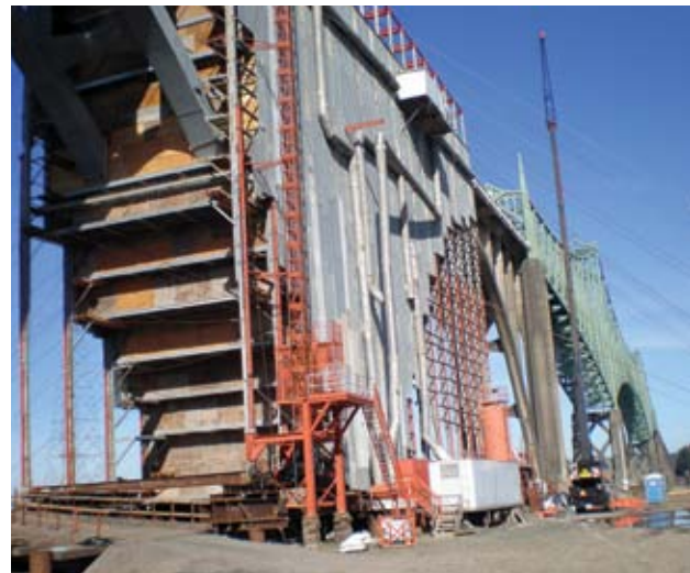
Up-close image of the enclosure showing a perspective of the size of the bridge and complexity of the project. The enclosure is roughly 100 ft (30.5 m) by 120 ft (36.5 m) long. Once the work inside is complete, the enclosure is dismantled and then moved down the line. At the end of the enclosure, you can see a stepping pattern as you follow from top to bottom. Each step represents a repair level—near the top there are “split levels”—16 total to address the complete structure
