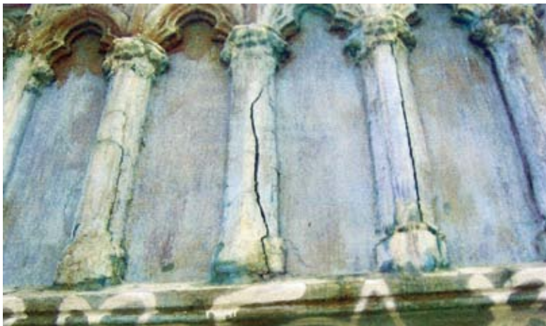
The spalled ornamental units created a dangerous condition
