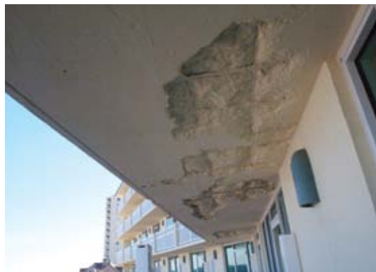
Severe underside spalling of balconies
