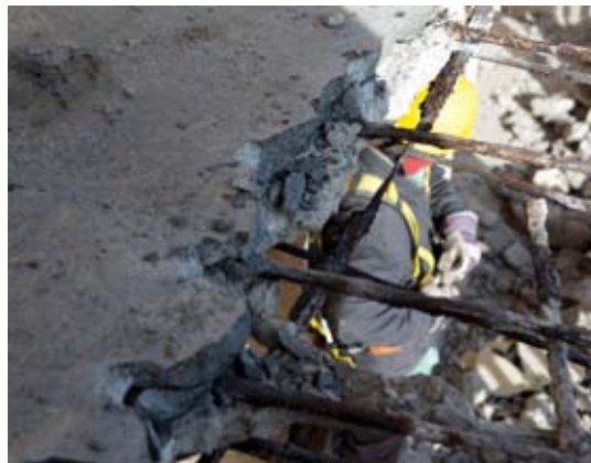
Reinforcing steel was extensively corroded
