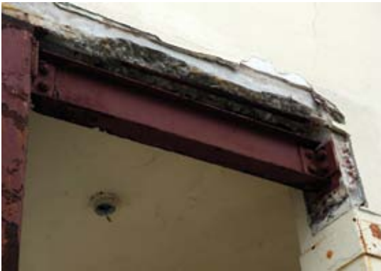
Corroded beams and columns were not capable of supporting loads much longer
