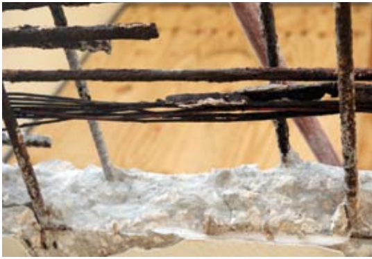
Close-up view of corroded reinforcing steel
