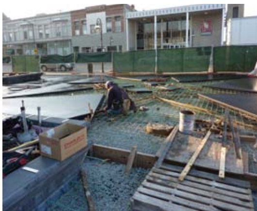
Installation of epoxy-coated reinforcement and intricacy of forming the integrated design features in the color concrete plaza slab
