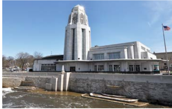
Overall view of completed river wall repairs, including rebuilt fishing platform, fountains, precast concrete stair, and precast concrete parapet walls
