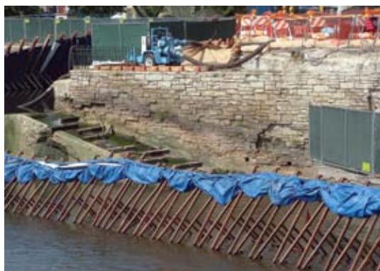
Extensive deterioration to the Lannon limestone cladding and underlying concrete wall at the north end of the river wall. Installation of the portable dam system for the contractor to perform repairs within the river is shown in the foreground
