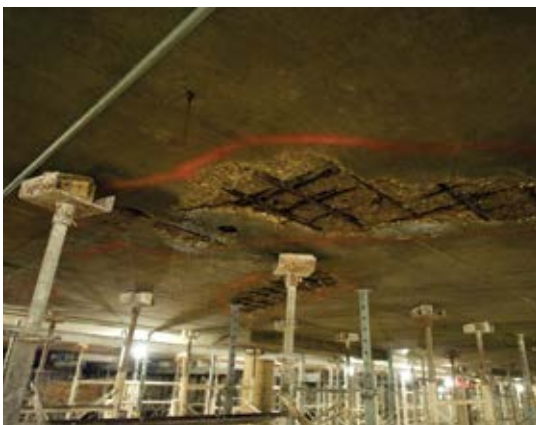
Deteriorated soffit areas identified for repair
