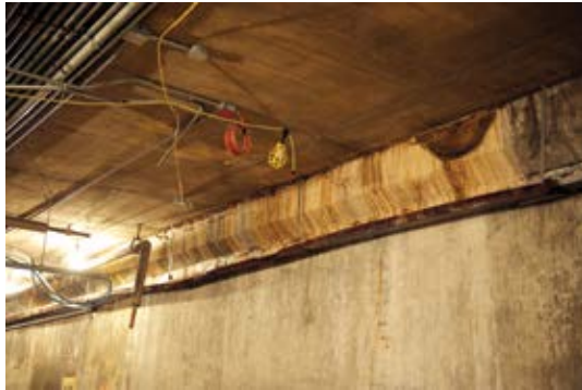
Deteriorated corbel area
