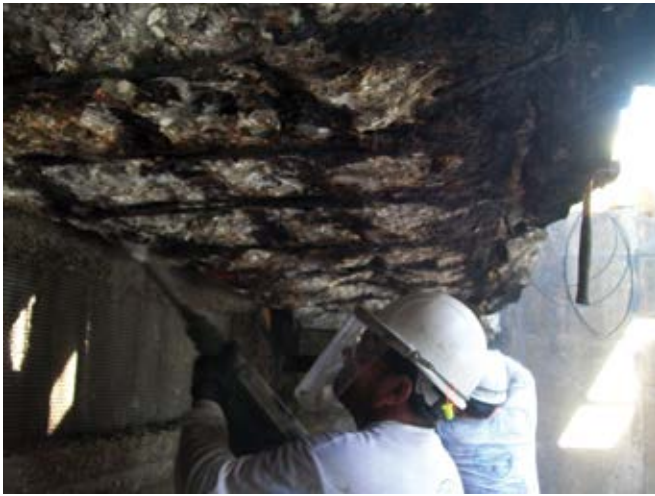
Workers chipping deteriorated concrete. Note complete loss of reinforcing steel
