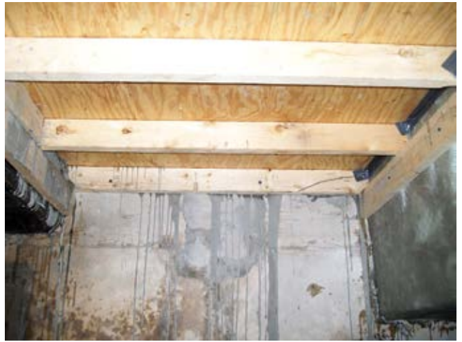
View of overhead deck repair with forms in place for pouring repair mortar
