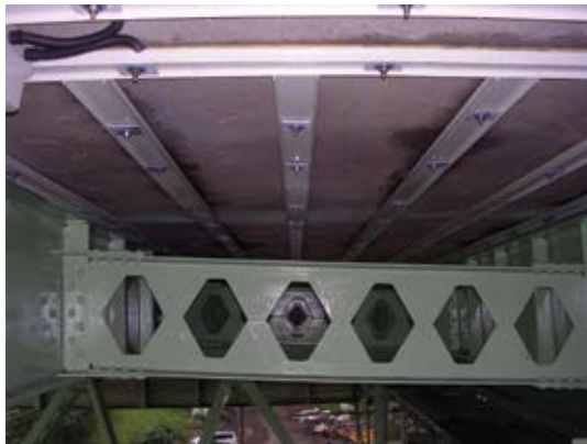
Installed cathodic protection "cassettes"
