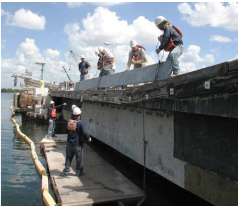
Work was difficult, as it had to be performed from the water
