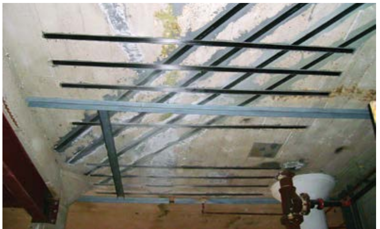
Fig. 5: Locations where original stresses were exceeded were reinforced with carbon fiber-reinforced polymer (CFRP) strips externally bonded to the slab with epoxy
