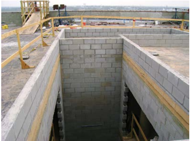
Fig. 3: At new service core openings, supplemental support for the slab was provided by new 6 in. (152 mm) load-bearing masonry walls around the perimeter of the shaft(s)
