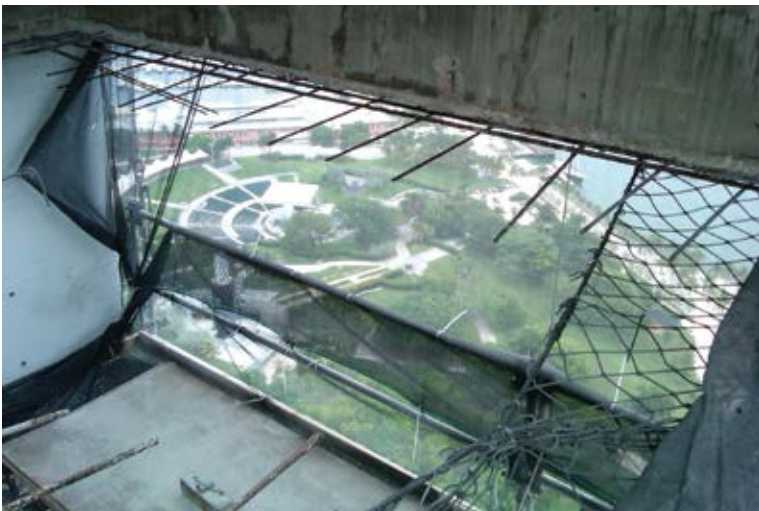
Cantilevered soffit slab after demolition, looking down to Bayfront Park and the bay
