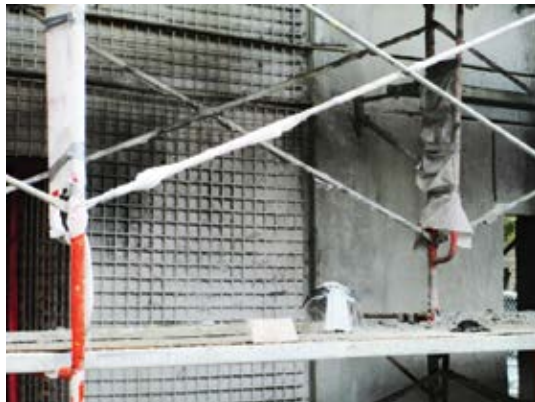
Fig. 6: A ferrocement coating provided lateral reinforcement to the CMU backup wall and provided a uniform finish to the interior of the park walls
