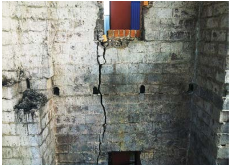
Fig. 3: A large crack that ran from the base to the top of the 50 ft (15 m) brick veneer façade (adjacent to the pedestrian sidewalk) indicated imminent collapse
