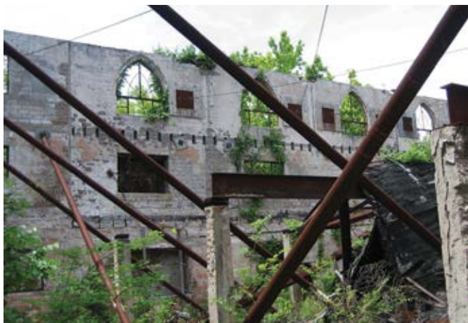
Fig. 2: Interior of gutted church
