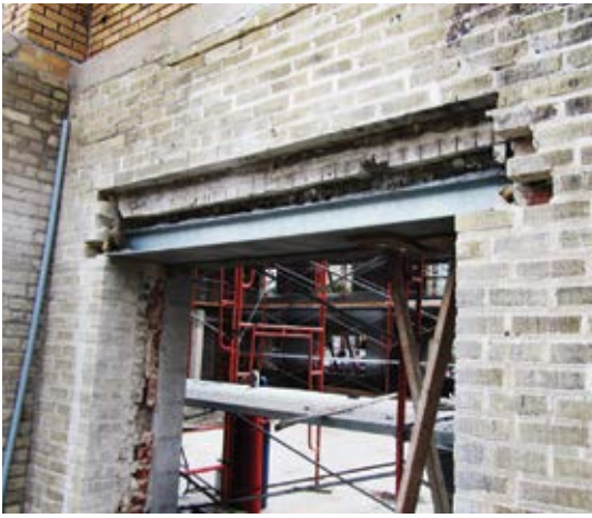
Fig. 8: Existing lintels over door and window openings in the 1923-era construction were removed and replaced
