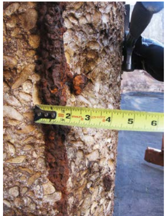
A typical view of embedded metal corrosion
