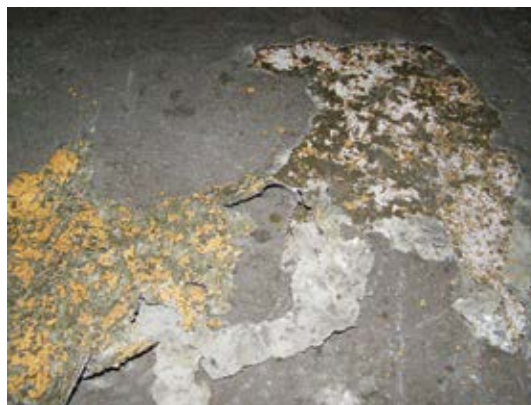
Failed coating and concrete
