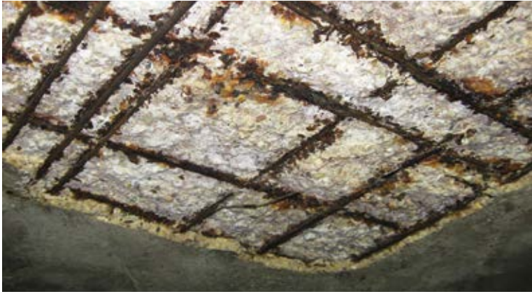
Overhead spall and corroded reinforcing steel
