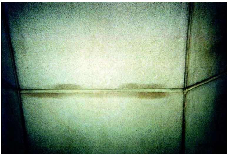
Figure 4: Stains on newer limestone panels below the third floor of the E Building
