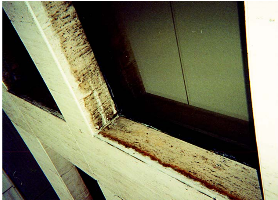
Figure 2: Dirt accumulation and staining of the D Building travertine
