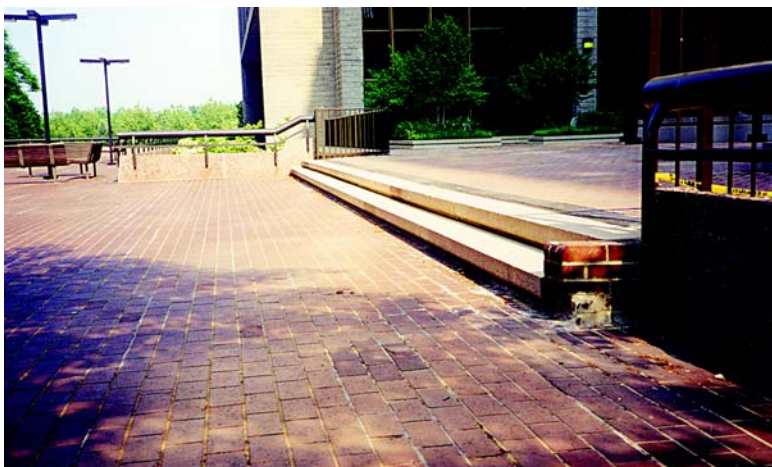
Fig. 1: Waterproofing membranes on concrete structures may be concealed by pavers, steps, masonry walls, planters, and many other coverings
