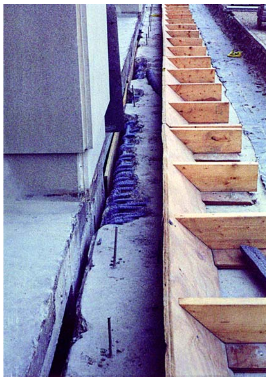
Fig. 5: Exposing the underlying concrete structure can reveal deteriorated concrete conditions
