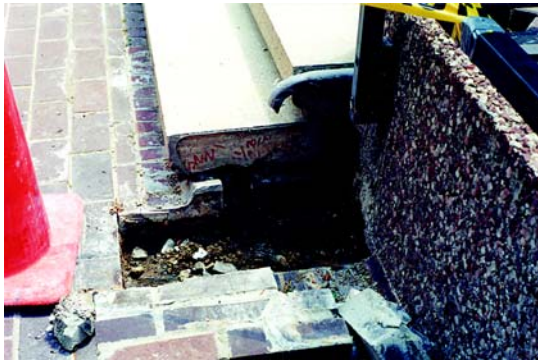
Fig. 3(a) and (b): Test holes should be performed at flashing detail locations, such as deck drains, perimeter walls, and transition areas (steps)
