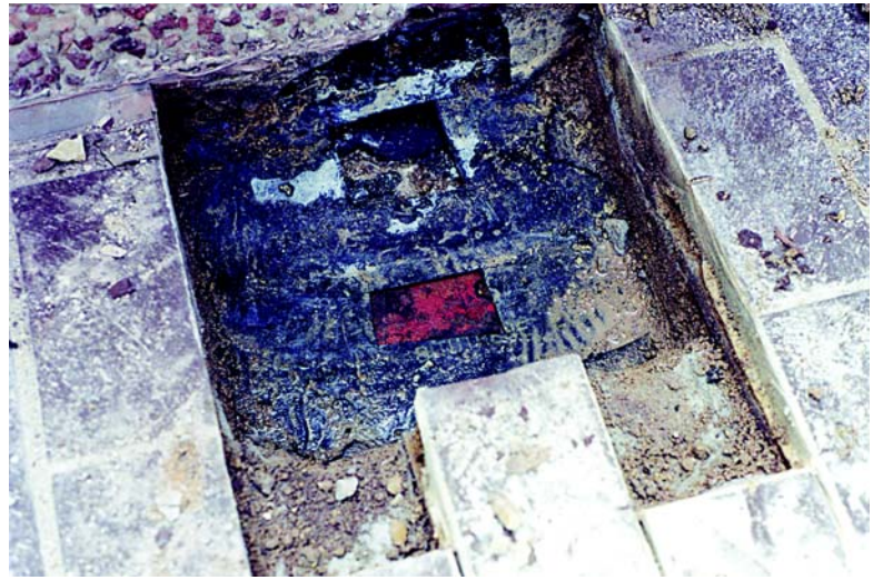
Fig. 4: Test cuts in the membrane assist in determining the existing condition and estimated remaining useful life of the membranes
