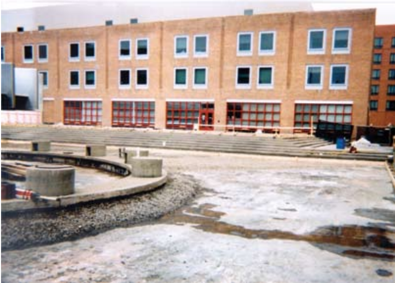
Lower level surrounding the fountain after demolition of existing exposed aggregate topping and removal of the existing gravel
