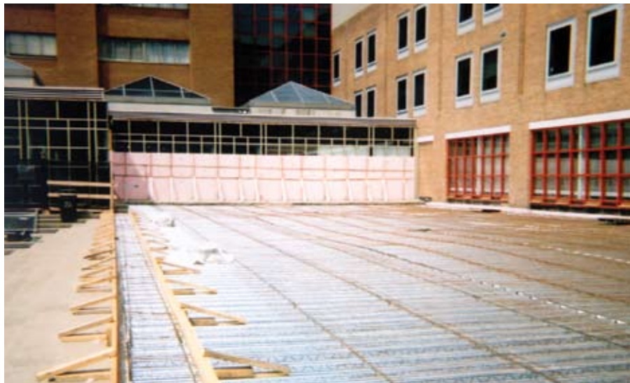
New composite pan deck on upper level prior to concrete placement, waterproofing, and paver placement
