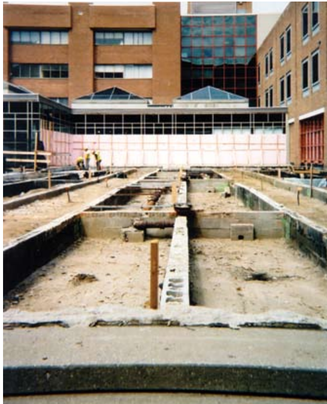
Upper level after demolition of existing exposed aggregate concrete topping and steel pan deck. Notice the 3 ft (0.9 m) CMU block wall cavities that were originally designed to raise the upper level above the other two levels. These block walls were repaired and heights were adjusted to allow for the new composite pan deck slab to slope to new drains slated for installation
