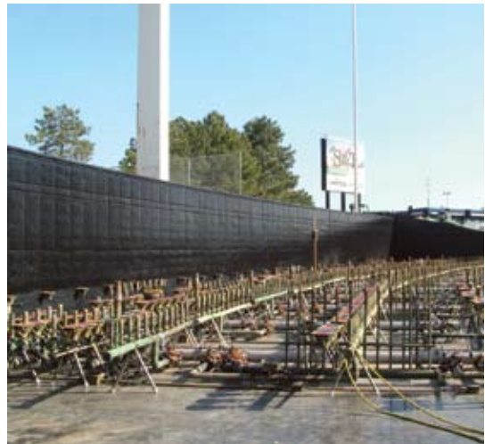
Main fountain: completed waterproofing membrane system and equipment installation in the upper pool area
