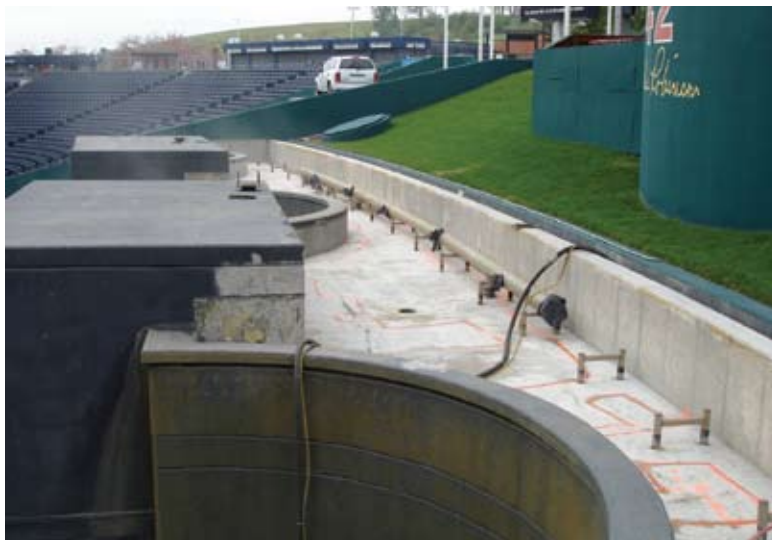
Secondary fountain: mapped out delamination locations
