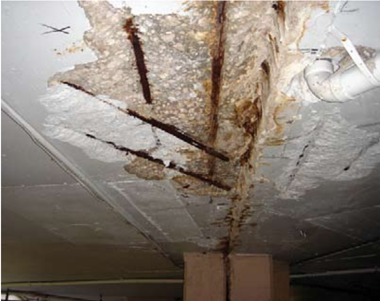
Fig. 5: Corroded steel in 440 West Condominium
