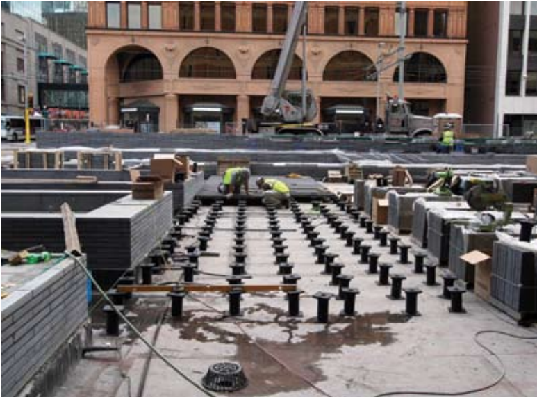
To allow future maintenance and inspection of the waterproofing systems, a pedestal system was installed for the new granite pavers
