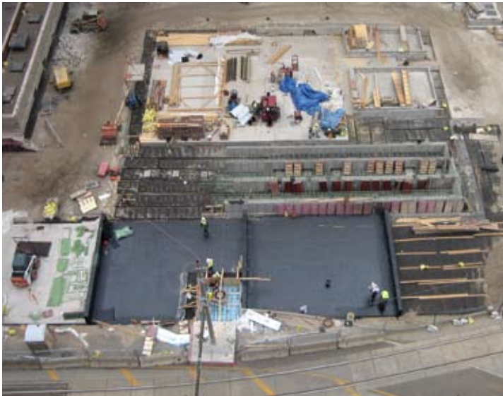
Waterproofing work began on the transformer vault portion of the plaza. Below the plaza is the key electrical transformer station for downtown Minneapolis businesses
