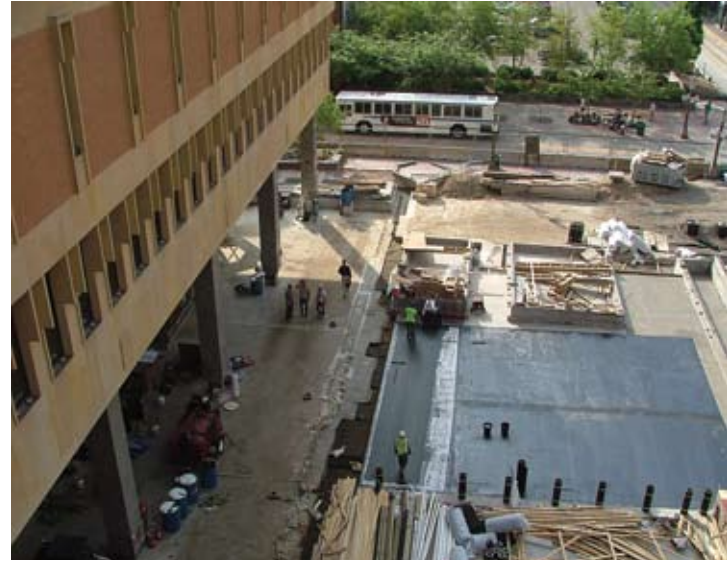
Once demolition was completed, waterproofing operations began. Careful planning and coordination allowed work to move forward with few glitches
