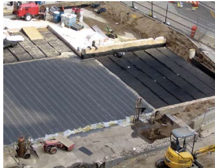
A high-performance waterproofing system comprised of multiple layers of hot-applied rubberized asphalt membrane and fabric reinforcing was applied
