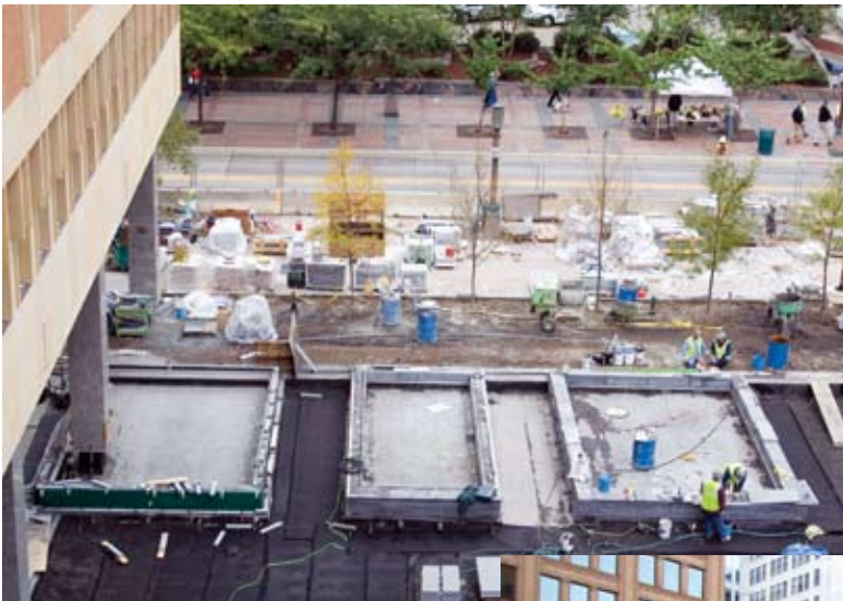
A goal of the plaza reconstruction was to protect the vulnerable transformers below, but also to create a welcoming space for pedestrians. Several new landscape planters were installed as a result
