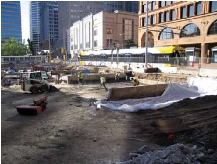
One side of the plaza is bordered by the new LRT system, which also includes a passenger stop. To complicate the waterproofing work, portions of the electrical power poles had to be temporarily rerouted and the roadbed stabilized, all with minimal disruption to the LRT
