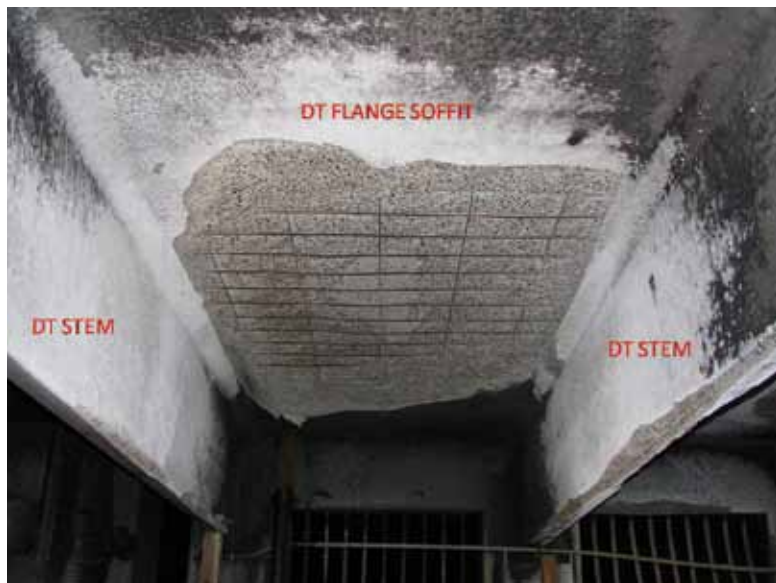
Fig. 1: Double-tee flange soffit and stem affected by the fire
