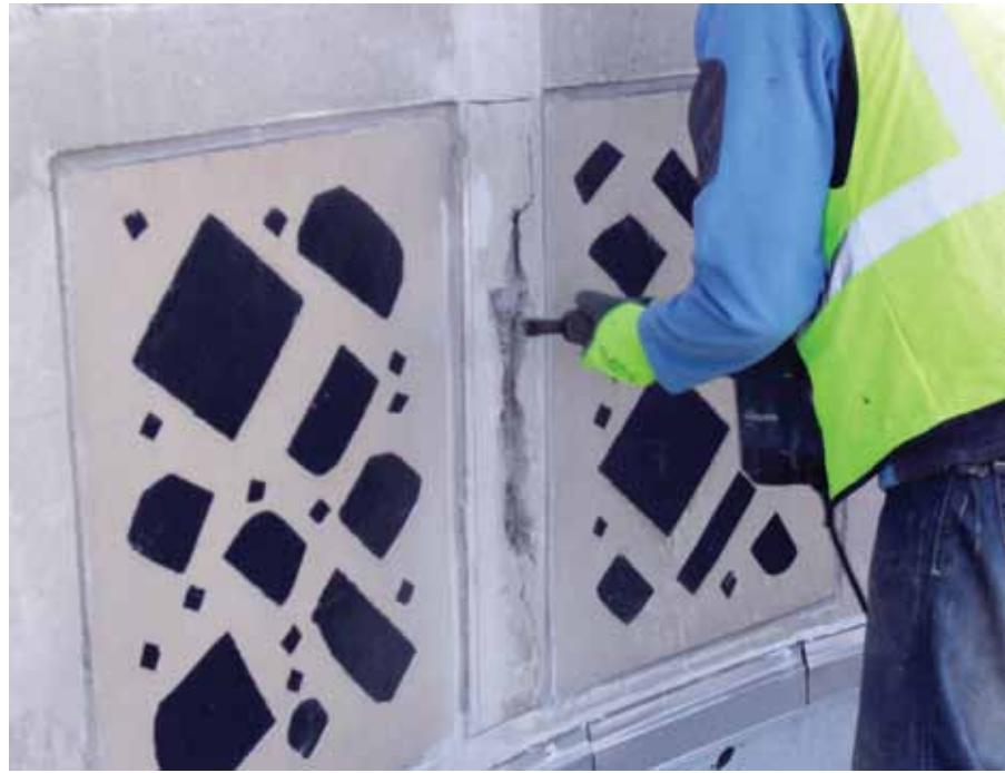
The first step was to chip out delaminated concrete until sound concrete was reached
