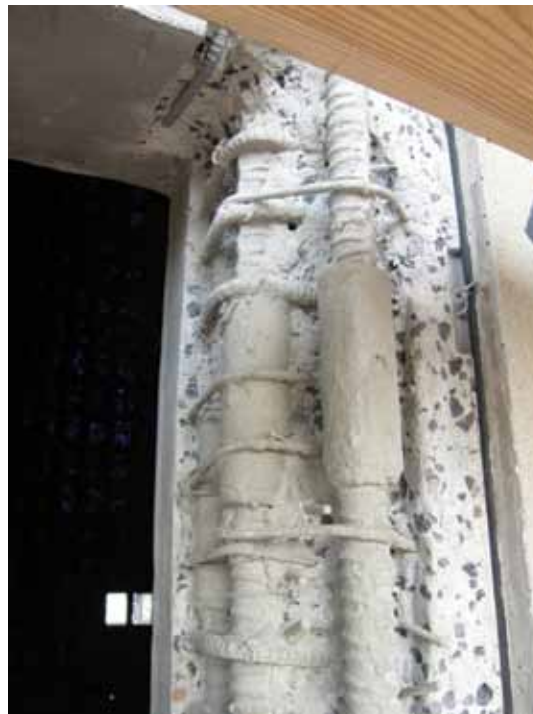
Once the steel was cleaned, it was immediately primed for corrosion protection
