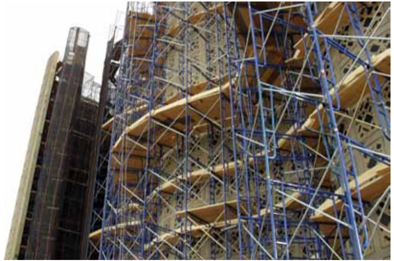
Because of the abnormal shape of the building, the scaffolding frames were kept a few feet away from the building and outriggers were used to butt up against the building
