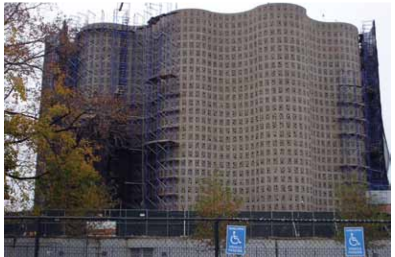
Fencing was installed around the perimeter of the structure; areas outside, however, were open to visitors and constant monitoring was required to ensure their safety
