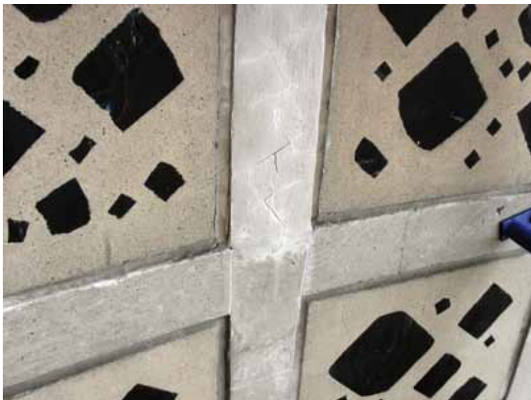
Deterioration could be seen at various spots on the building, mainly due to inadequate reinforcing steel coverage
