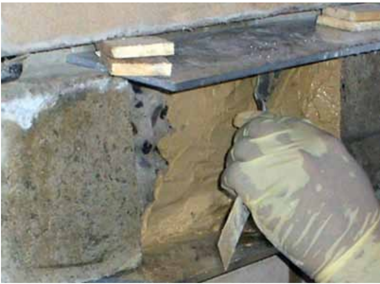
To ensure that the sides of the patches stayed square and in line with the existing substrate, small pieces of methylmethacrylate were set in place to give applicators a side edge for the patch
