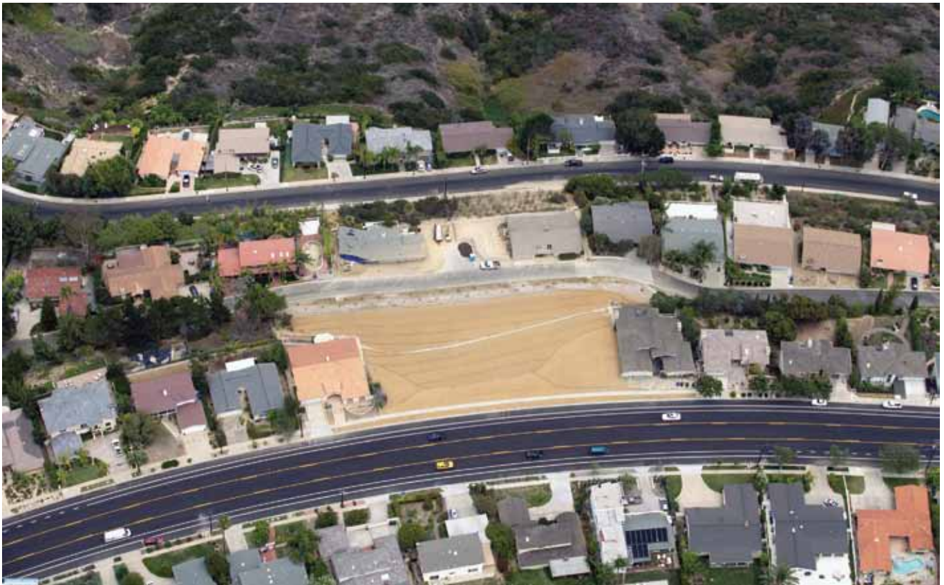
Completed landslide remediation repair of Soledad Mountain Road and Upper Desert View Drive
