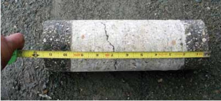
Fig. 5: The core with a crack in the grout
