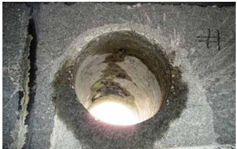
Fig. 2: View of the core hole showing honeycombing of the grout on the upper portion
