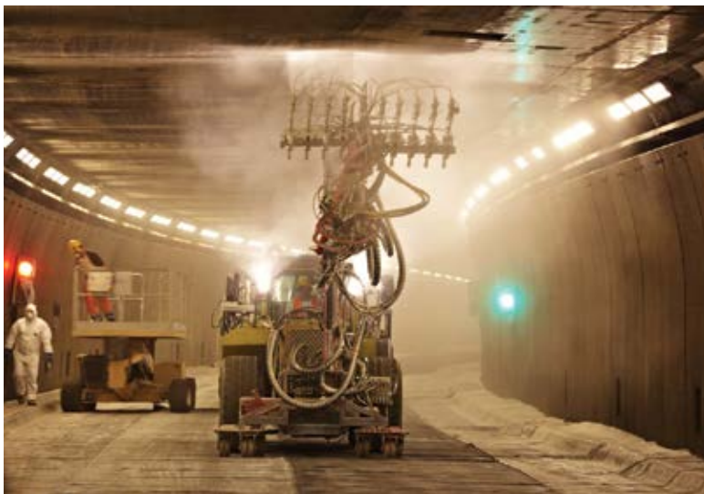
Fig. 8: Silane cream applied at the crown of the Gotthard tunnel in Switzerland. 64,600 ft 2 (approximately 6000 m 2 ) were treated overnight with airless spray application
