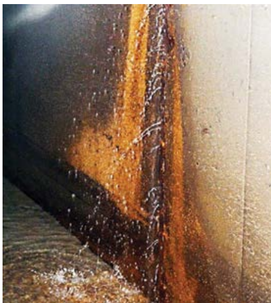
Fig. 4: Active leak in common wall
