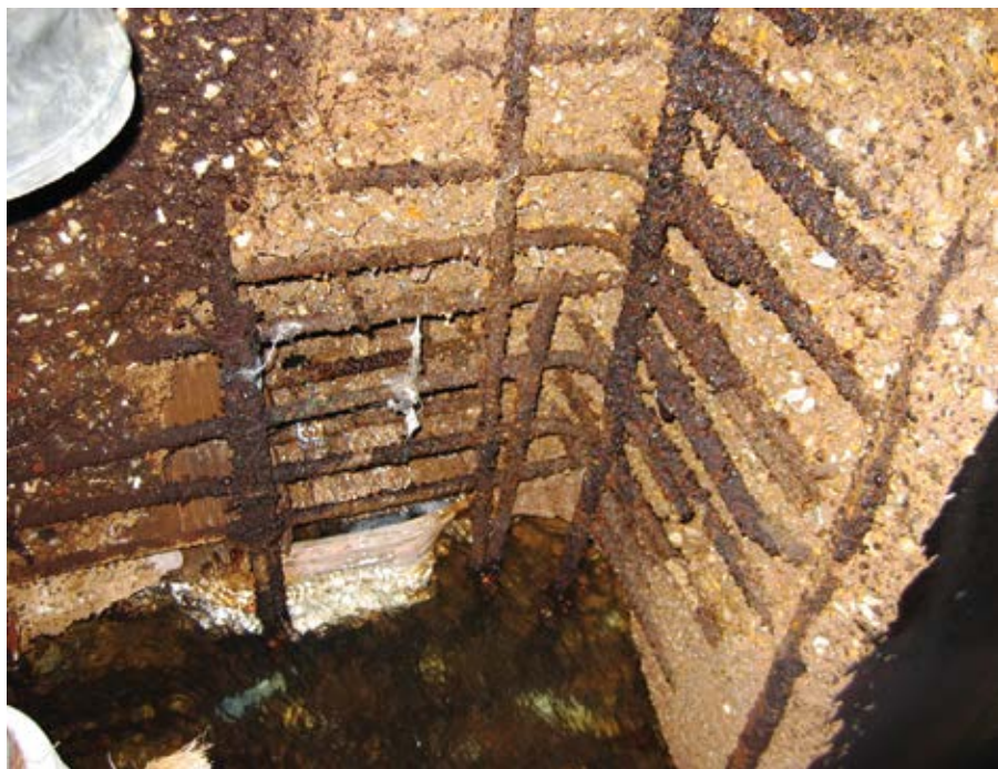
Fig. 2: Severe concrete and reinforcing steel deterioration due to hydrochloric acid exposure
