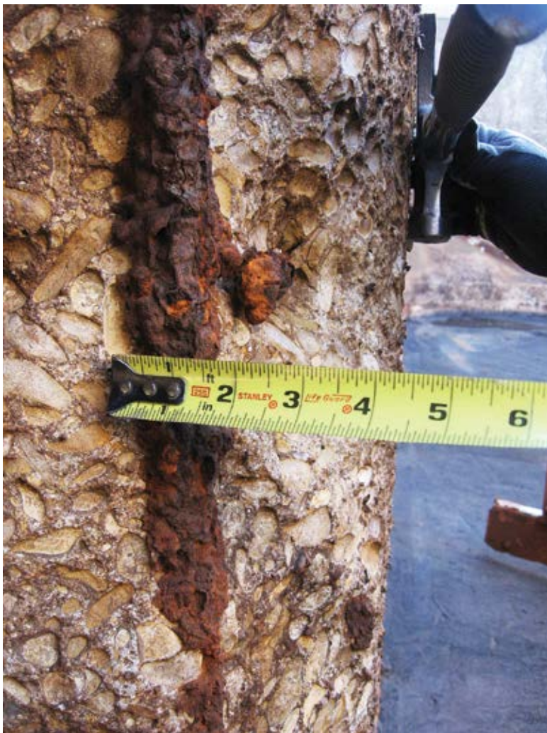
Fig. 1: Severe concrete matrix loss and corrosion of underlying reinforcement due to carbonation
