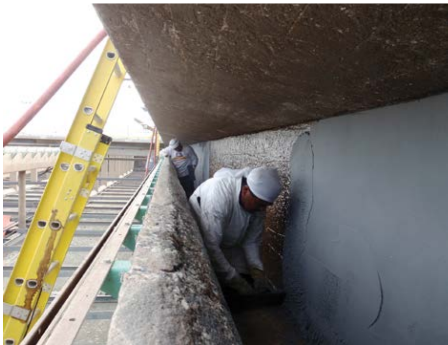
Fig. 4: Application of epoxy-based, quartz-reinforced composite overlay on the effluent trough of a clarifier basin
