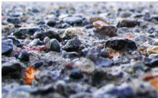
Fig. 1: Surface prepared using hydrodemolition has a rough, irregular profile with protruding aggregate essential for creating a mechanical bond
