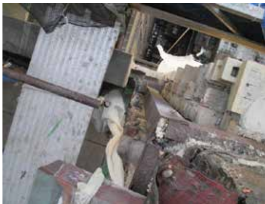
Fig. 4: Looking down at the twisted corner column shown in Fig.3 resulting from the loads applied to the severely corroded column
