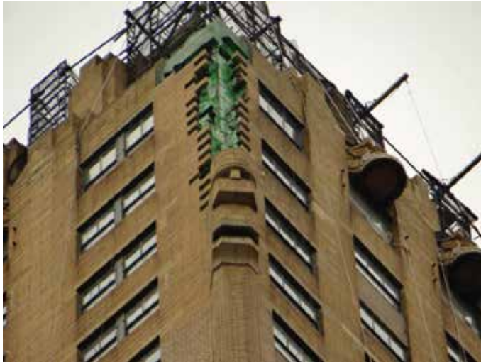
Fig. 7: Demolished, prepared and waterproofed corner from the 50th to the 53rd floor at the southeast corner of the tower
