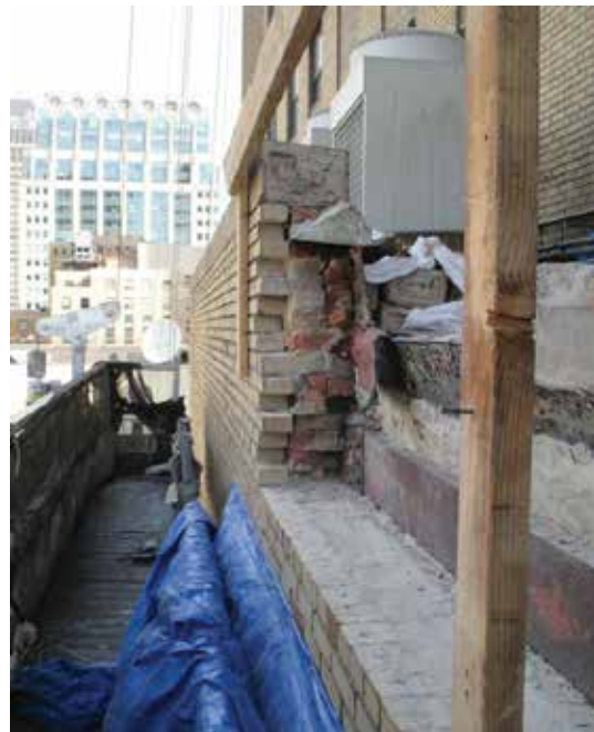
Fig. 5: View of the west parapet wall of the 32nd floor setback on the west elevation, where there is no lateral reinforcement of the parapet due to the corrosion from water penetration through the parapet masonry with poor original construction and prior roof leaks before the roof was replaced in 2007
