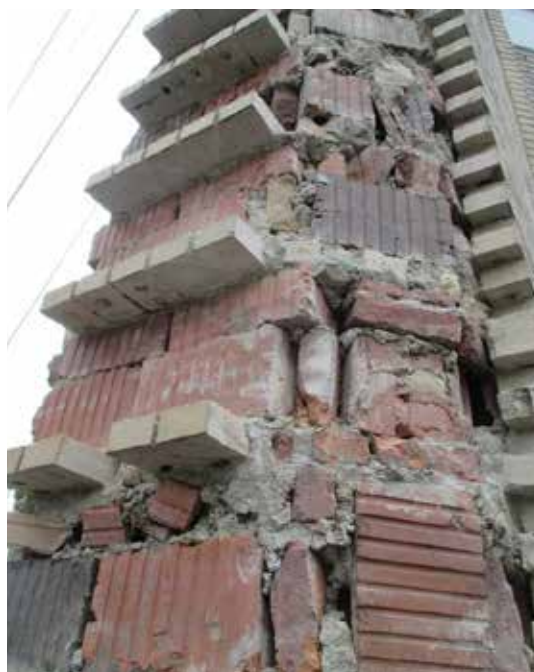
Fig. 2: View of the 32nd floor northeast fin (corner) with the face brick removed and backup masonry exposed
