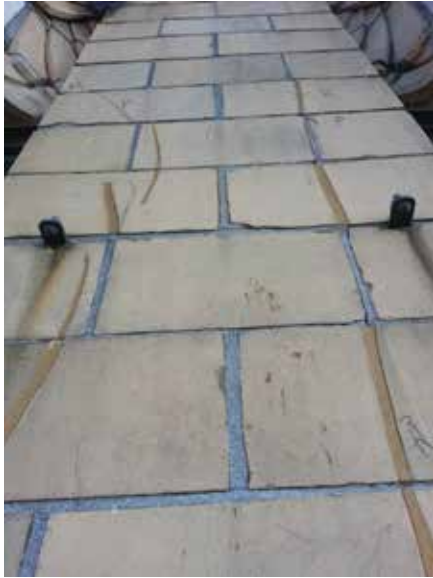
Fig. 6: View of 2nd pier from the east on the south elevation at the 52nd floor with severe and repeated cracking of the terra cotta and repair mortar
