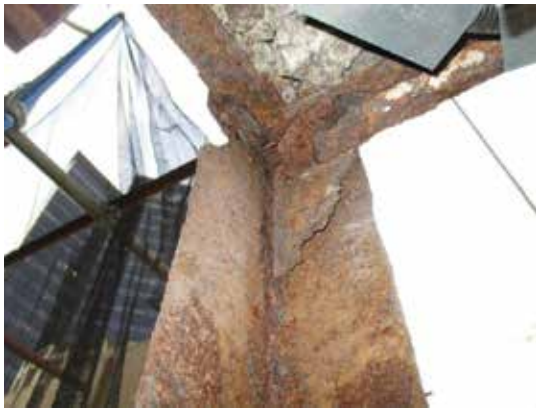
Fig. 3: Southwest corner of 32nd floor setback on the west elevation where water penetration from the roof and through the masonry resulted in the column corroding (the column and roof channels were replaced)
