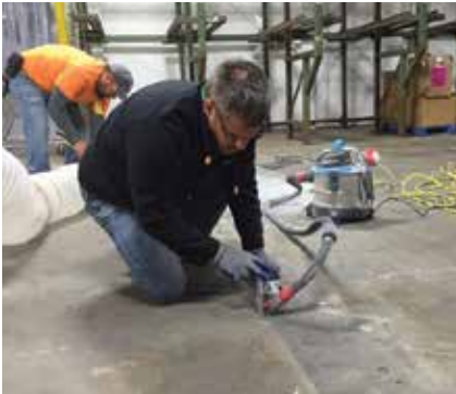
During the Spring Conference, the chapter also completed its annual Service Project, providing repairs to a cracked concrete floor at the Harvest Hope Food Bank in Greenville, SC
