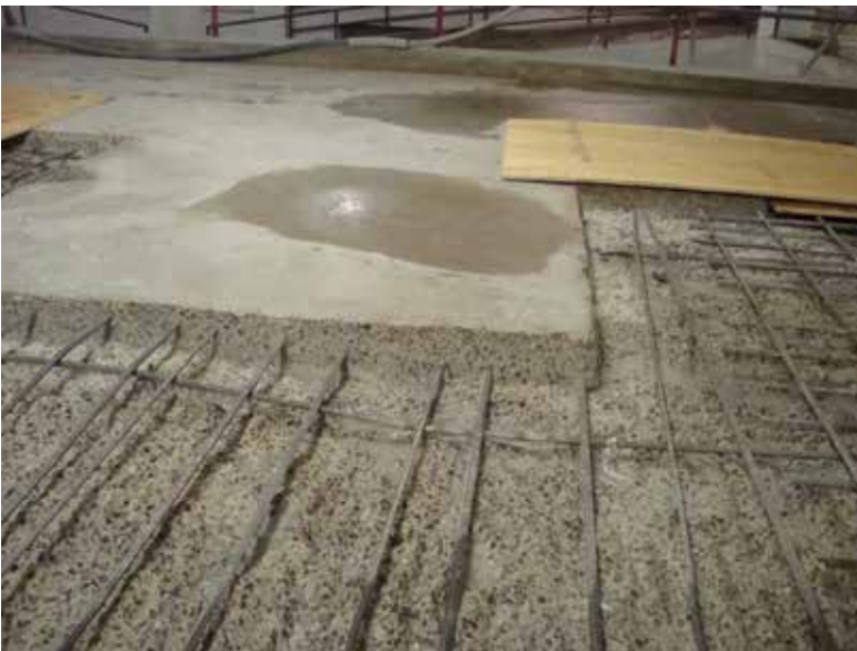
Fig. 7: Varying depth of concrete removal due to improper bar placement
