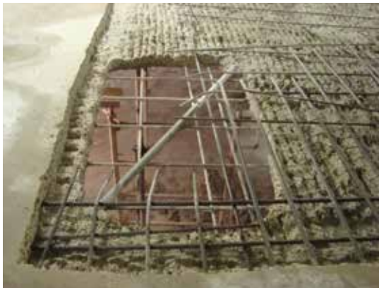
Fig. 8: Sound metal conduit undamaged from hydrodemolition
