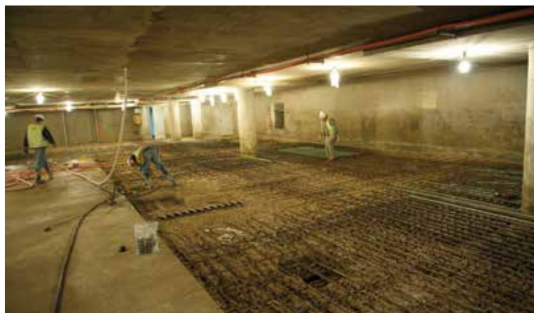
Fig. 2: Hydrodemolition provides superior surface preparation of existing concrete and reinforcing steel surfaces
