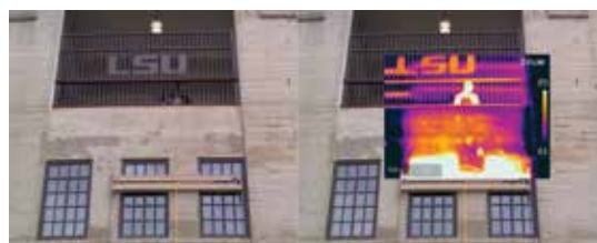
Fig. 2: Thermal imaging for concrete spall detection (before and after)
