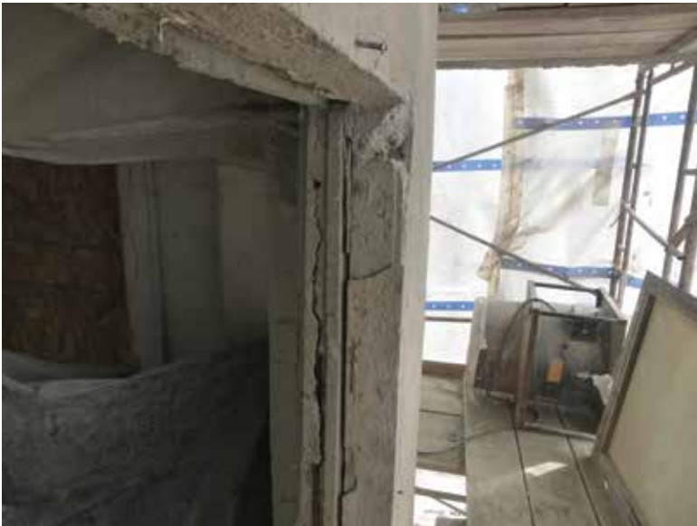
Fig. 6: Deteriorated concrete window jamb at facade of building. Note vertical crack at location of embedded steel angle from previous window frame (2014)
