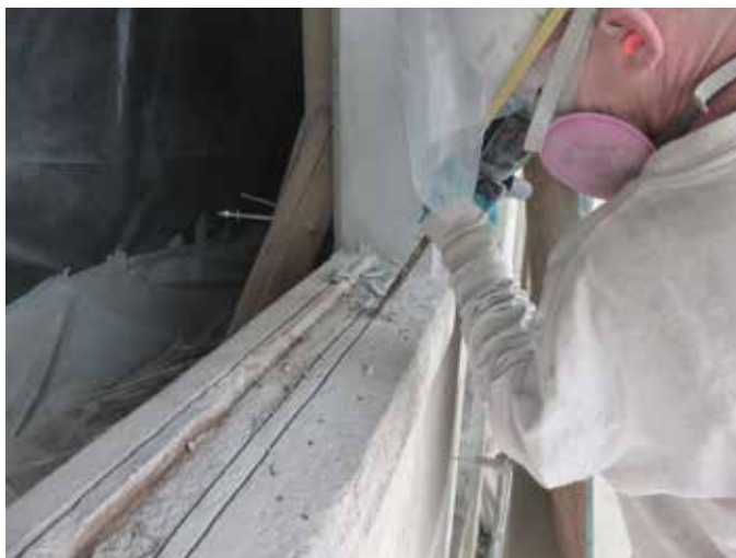
Fig. 8: Saw cutting and chipping of concrete sill to create recessed flashing ledge for new window sill (2014)
