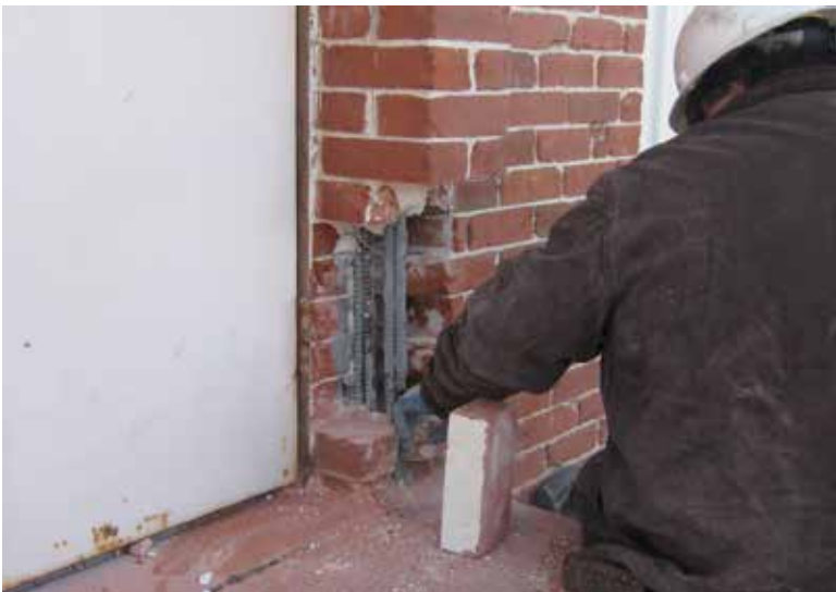
Fig. 5: Deteriorated brick and mortar replacement at masonry pilaster
