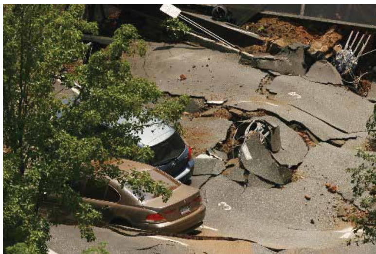
Fig. 3: Garage collapse due to reduced structural capacity
