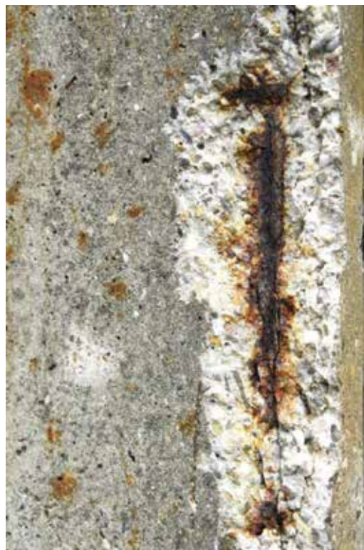
Fig. 2: Spalled concrete due to corrosion of reinforcing steel
