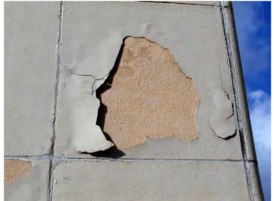
Failed Epoxy-Based Resurfacing Mortar
