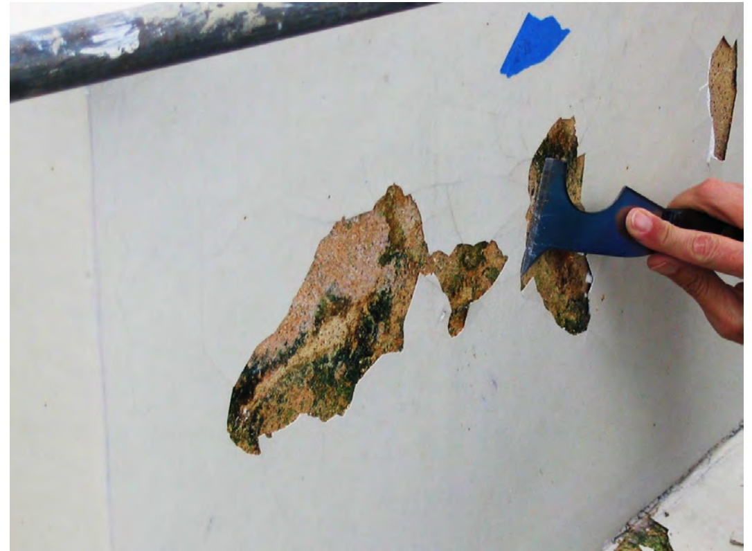
Biological Growth in Wet Bisque Beneath Spalling Glaze
