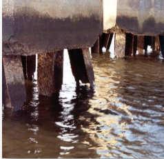
»Badly deteriorated H-Piles
