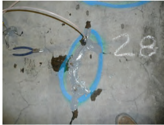
Fig. 2: Injection showing adhesive travel beyond the cap seal
