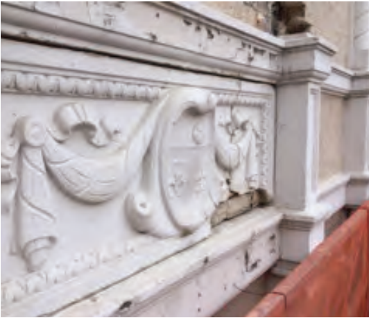
Fig. 2: Typical deteriorated façade spandrel panel
