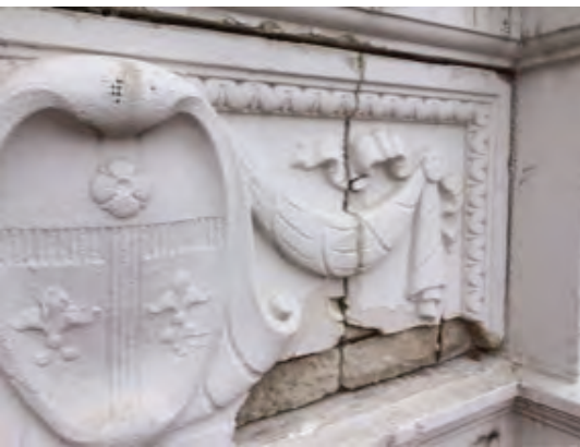
Fig. 3: Cracked and spalled cast stone at façade spandrel panel
