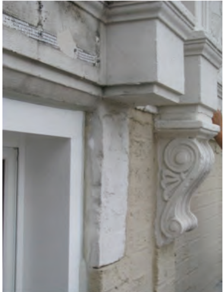
Fig. 4: Missing architectural façade bracket
