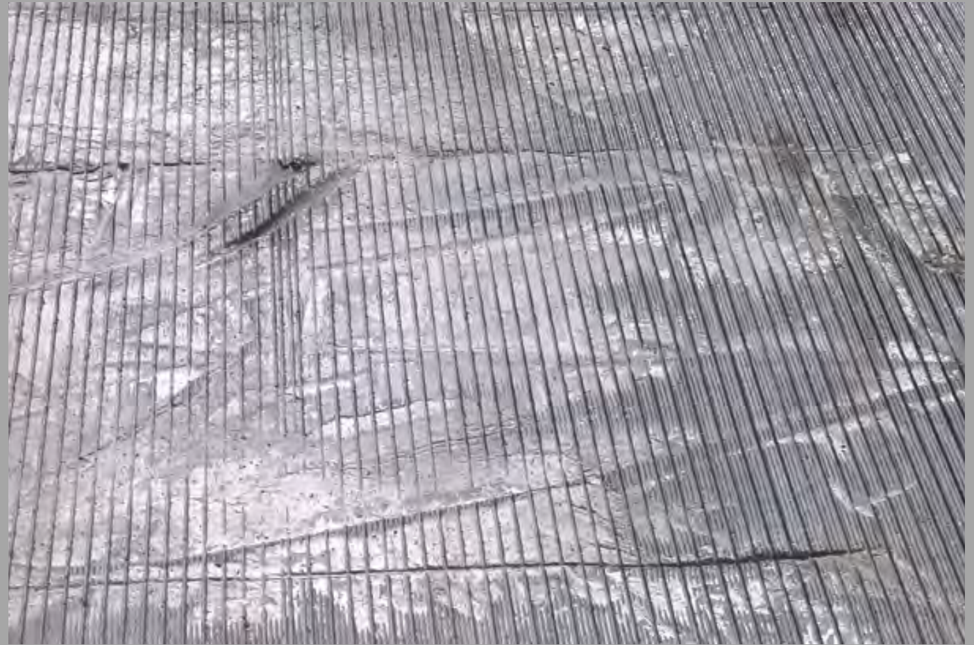
Impressions in final grinded and grooved surface from sheeting
