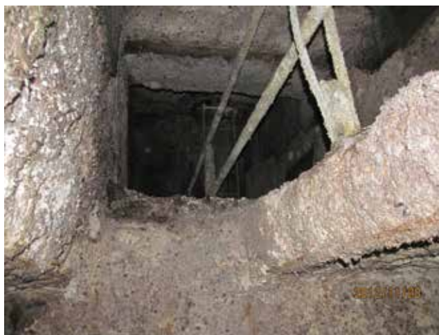
Fig. 4: Severe corrosion of metal railings above wastewater flow
