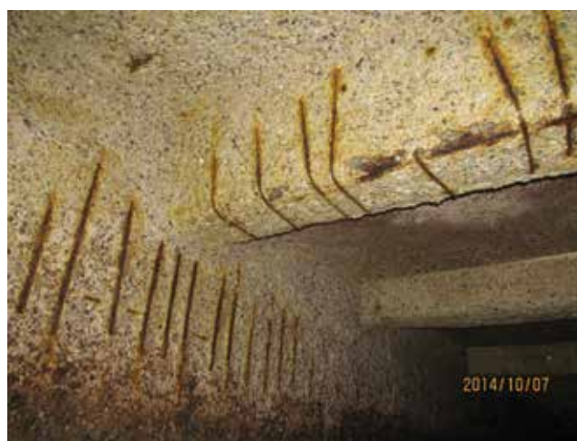
Fig. 3: Exposed reinforcing steel at beam and wall surfaces
