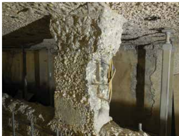
Fig. 2: Existing column deterioration
