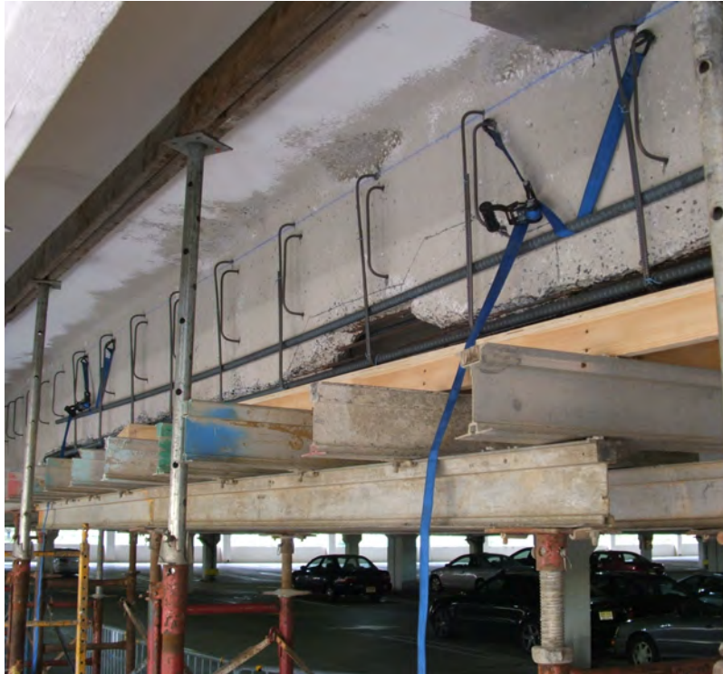
Buildout of damaged tee stem
