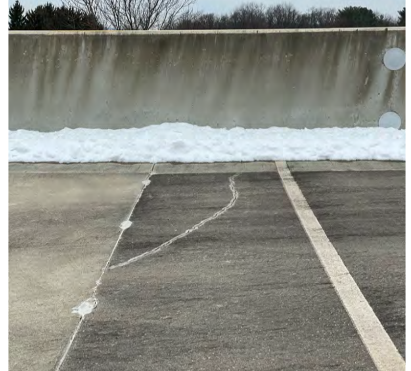
Cracked corner of tee flange
