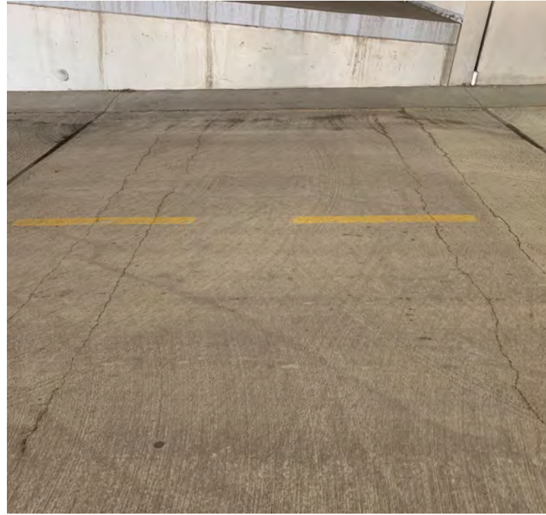
Cracking over each tee stem
