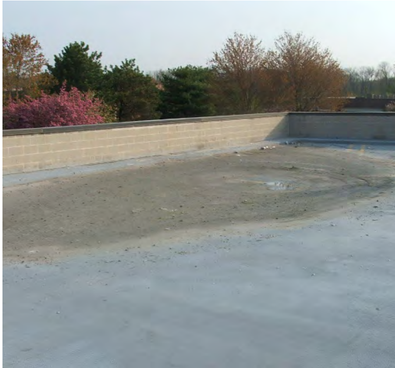
Deflection in area of beam failure
