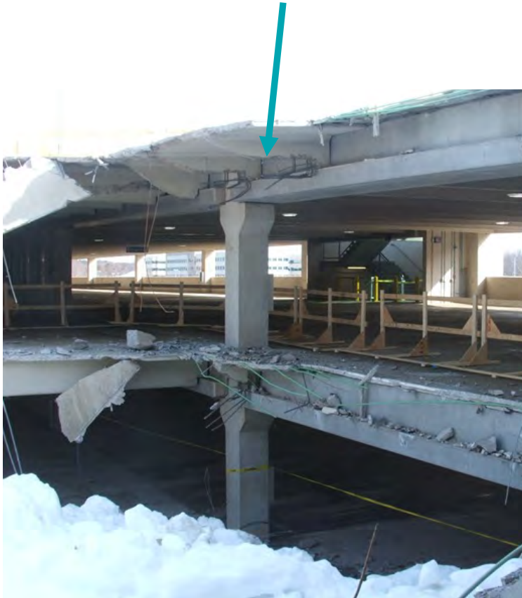
Shear failure of double tee stems
