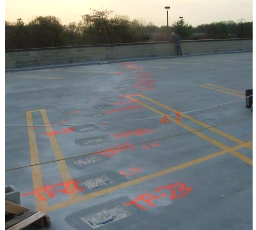
Broken tendons (full bay)
