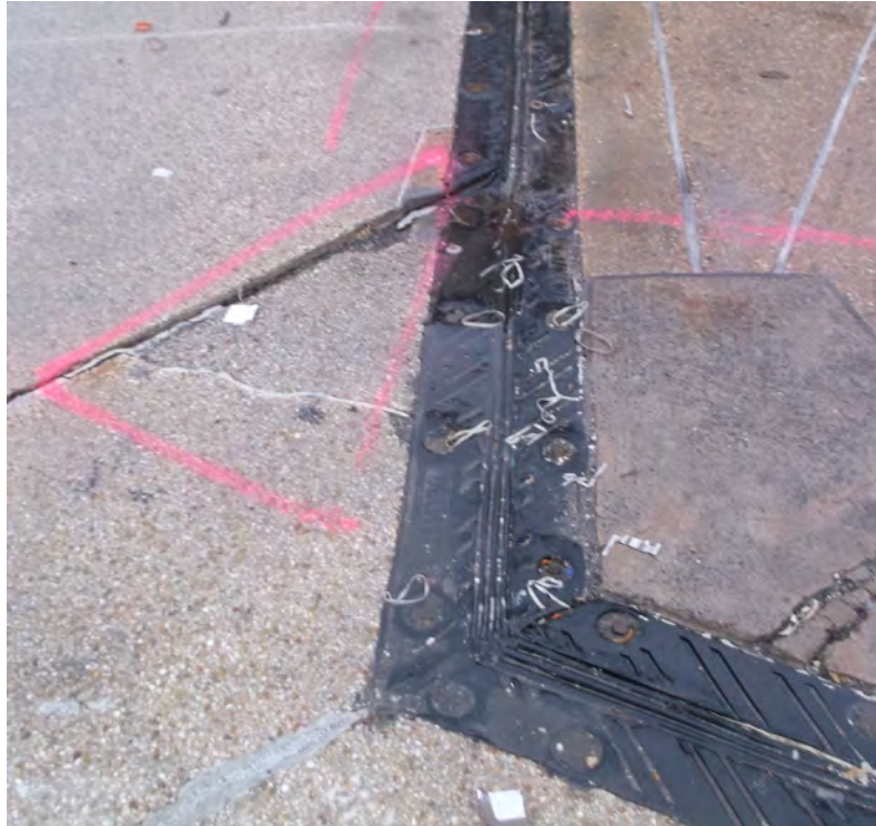
Cracked corner of tee flange
