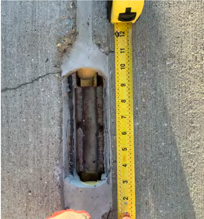
Broken shear connection and cracking of tee flange
