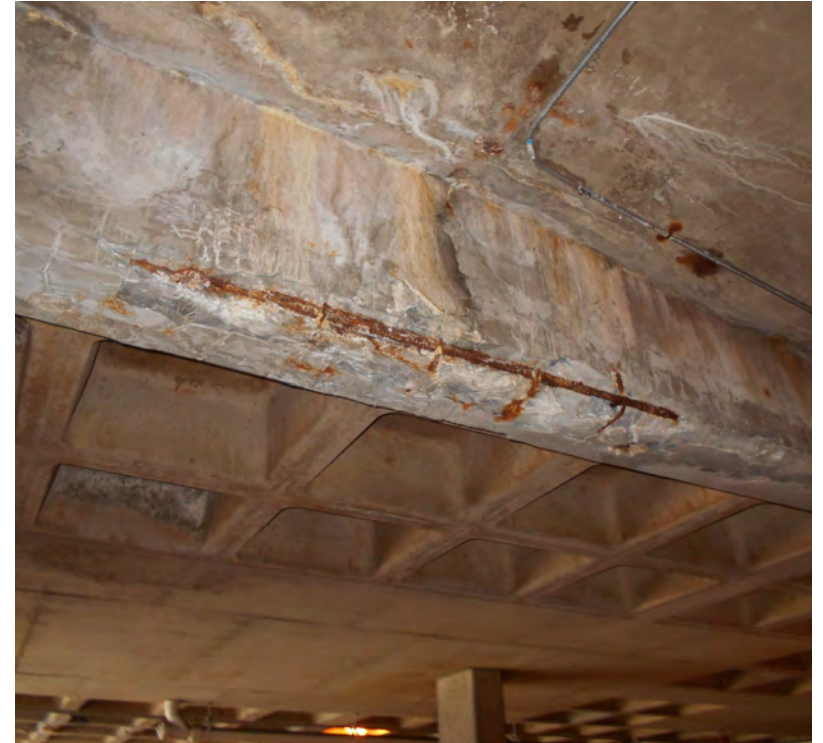
Cracking and deterioration in CIP beam
