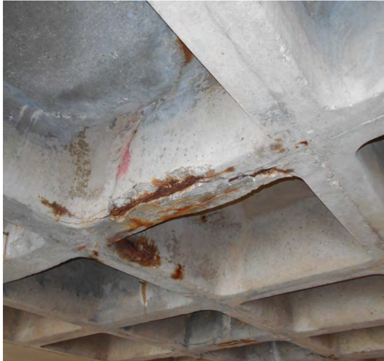
Cracking and deterioration in waffle slab
