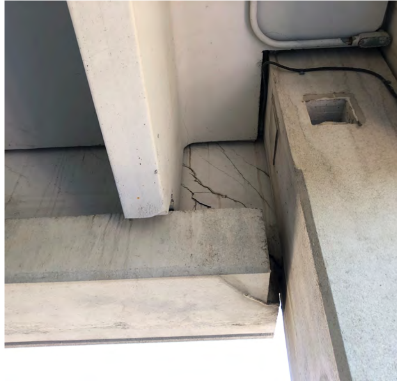
Shear cracking in spandrel panel
