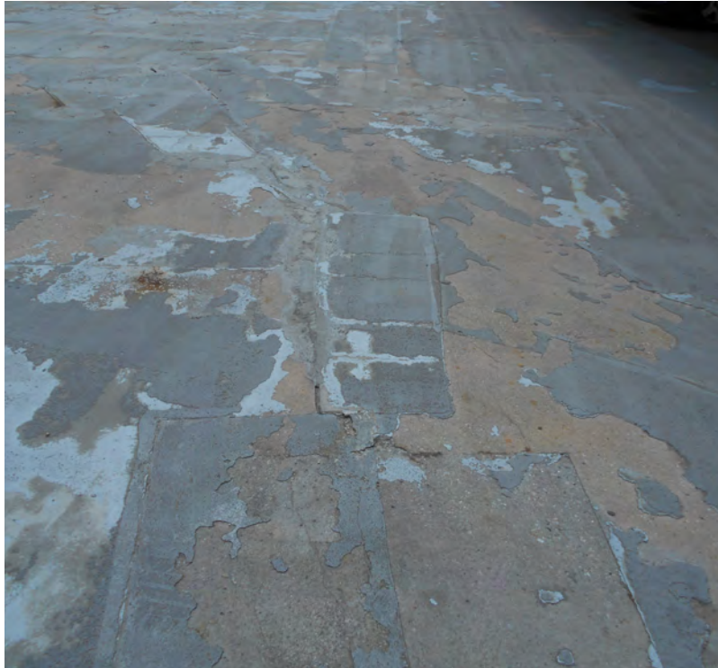
Cracking and deterioration in top slab
