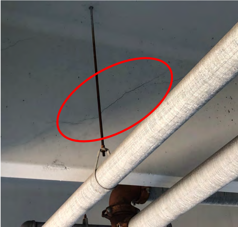
Shear cracking in tee stem
