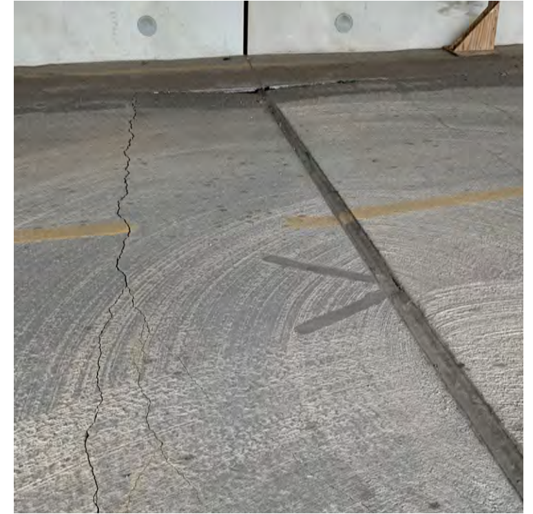
Tee flange deflection and broken connections at joint
