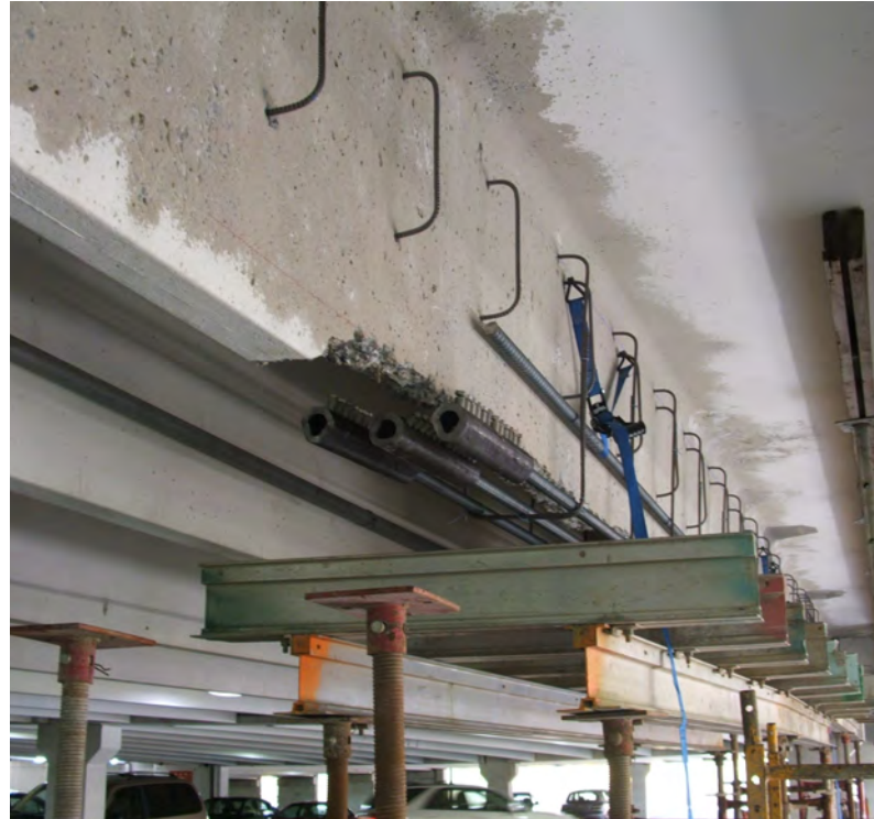
Buildout of damaged tee stem
